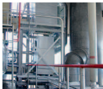
From left to right: Steam boiler with economiser and flue gas condenser, steam boiler before retrofit, flue gas condenser and economiser
