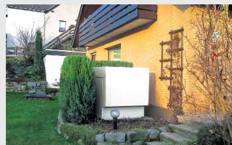
Air/Water heat pump placed outside
