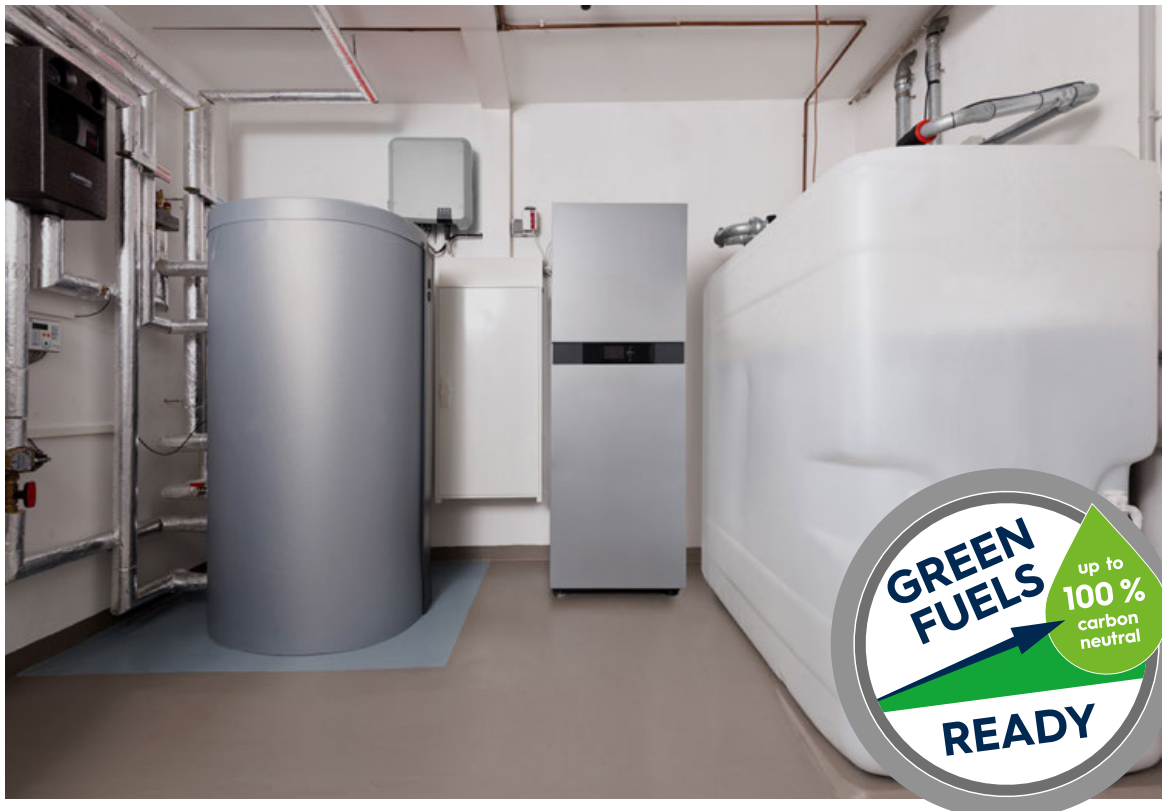
The energy stock in the tank ensures a reliable heat supply
